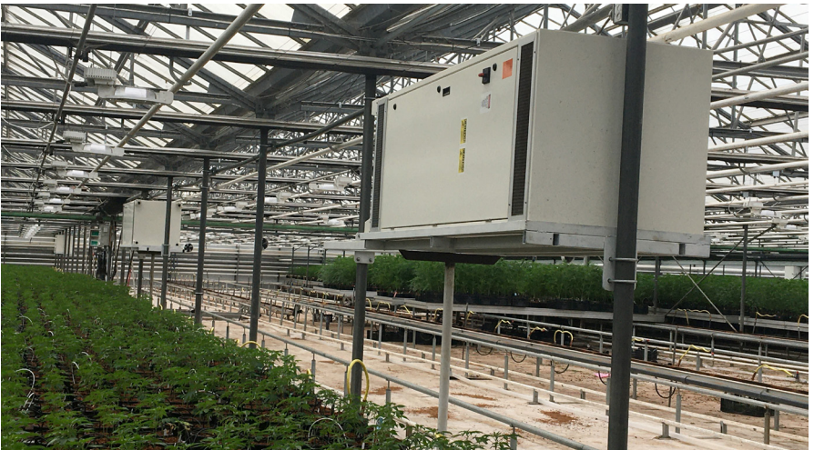
Envinity scrubbers from the Netherlands, shown here at Ever-Bloom, have been found to remove 84 percent of the smell of cannabis inside a greenhouse, on average. Photo by Melinda Burns.
